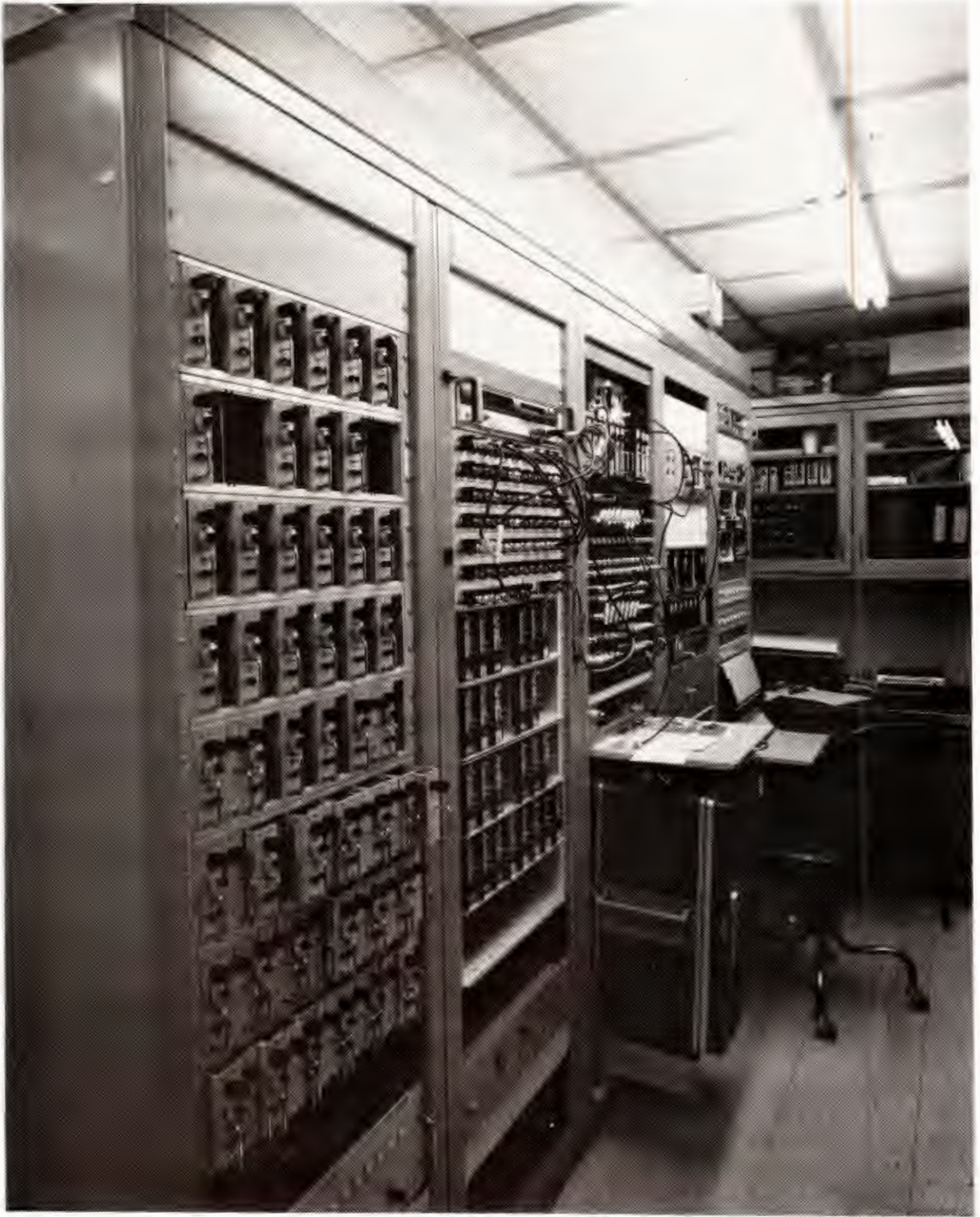
Fig. 13. Data acquisition system.
