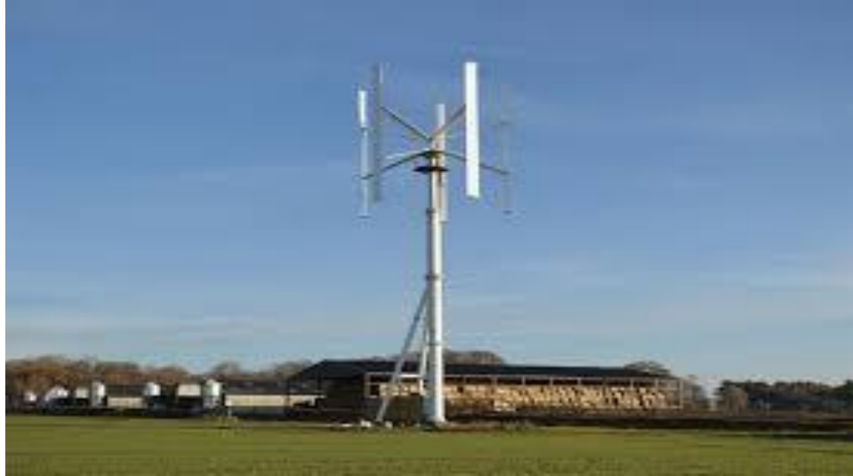
Figure 2. Vertical-Axis Wind Turbine
