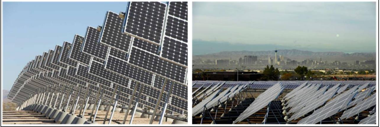
Figure 4. Nellis AFB Photovoltaic Solar Facility
